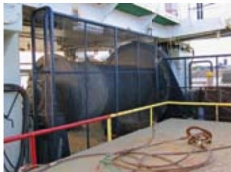
Protective safeguards around winches
