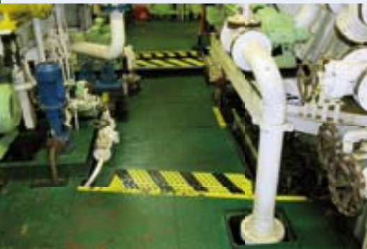
Extra step added in the engine room
