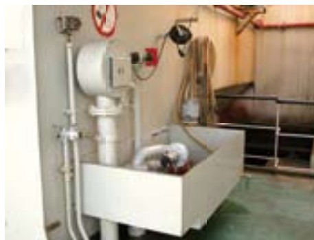
Drip tray around Winel tank vent
